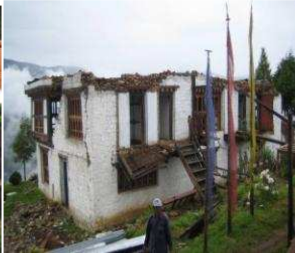
Narang: Seriously damaged dwelling
