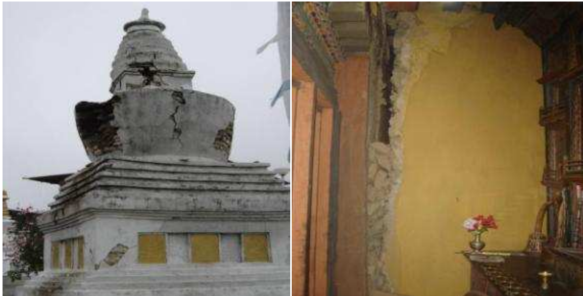
Drametse: Damaged Stupa and inner Monastery walls separating from wooden framework
