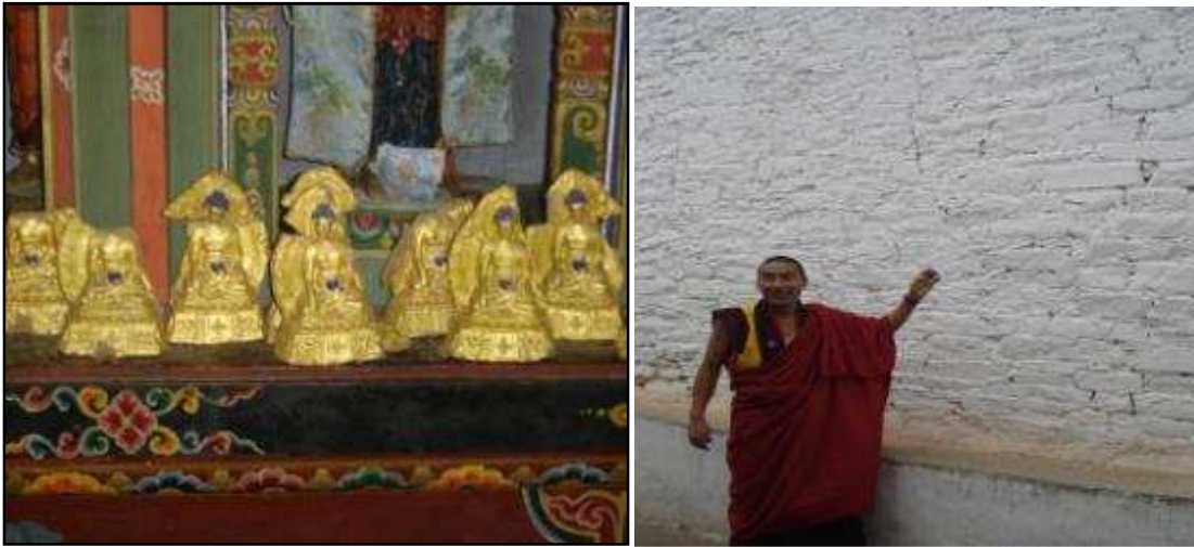
Drametse: Earthquake damage to inner statues as well as exterior Monastery walls
