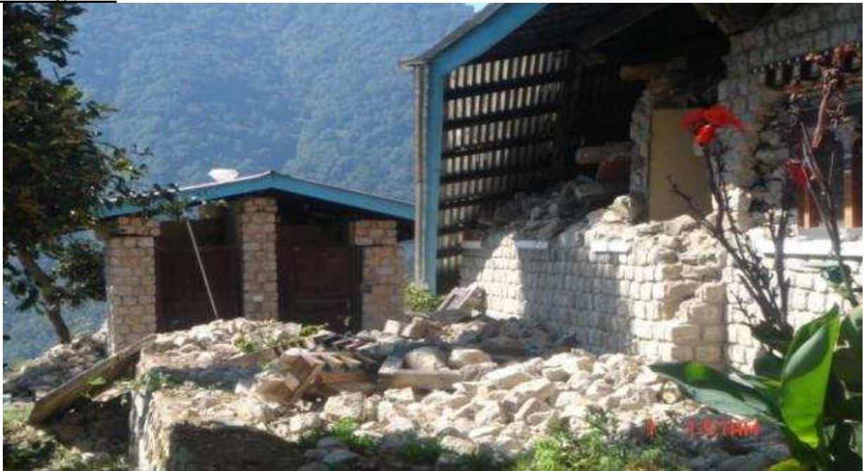
The Narang BHU Grade II buildings completed in 2007, consist of 4 buildings which have collapsed due to the quake.
