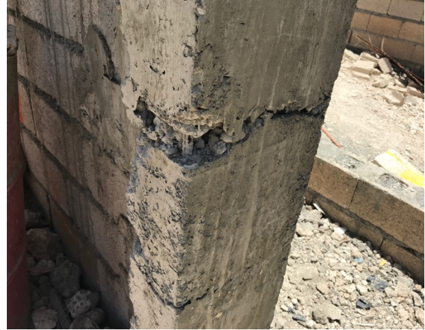
Photo 14: This photo shows the common result of bad concrete compaction. From another angle it also shows the tip of what is called locally an “earthquake” bar. These are horizontal reinforcement bars running along the bond of every 4 courses of block. These are tied to the vertical bars and inserted into the stiffeners.
