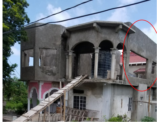
Photo 10: This second story is extremely vulnerable. Not only do the upper walls not align with the bottom walls but construction is extremely irregular and there are very few shear walls. The wall on the right of the building could collapse in high winds if not laterally supported soon.
