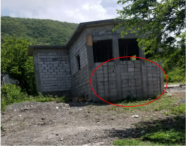
Photo 9: Blockwork quality varies significantly from site to site. Here is an example of block that hasn't been interlocked.
