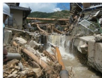
Photo 1. Exposed Distribution Mains after 2014 Landslides in Hiroshima
