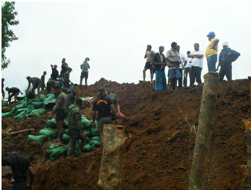
Figure 5.13 Landslide – Sri Lanka
