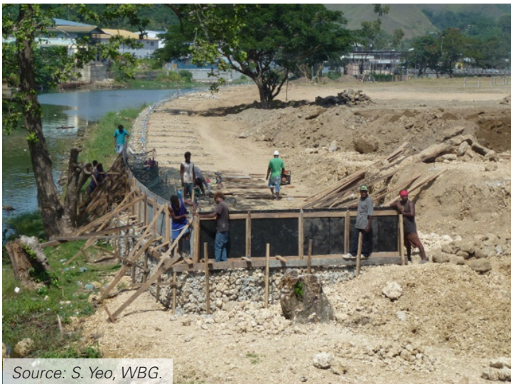
Figure 19. Filling the floodplain and riverbank protection works on one side of the Mataniko River in Honiara
